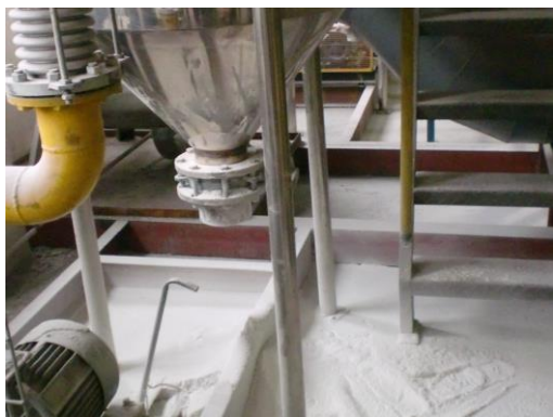
粉尘泄漏—整改前
